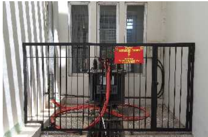
(b) Transformator Tenaga Listrik Step-Up
